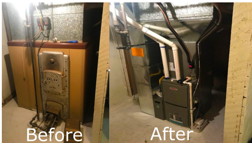
An example of a furnace replacement utilizing funds from a newly created program called the Crisis Program. The program provides funding for BRAG staff to repair furnaces for low-income households, and even repair or replace water heaters and air conditioners for seniors, persons with disabilities, or those who have young children.
